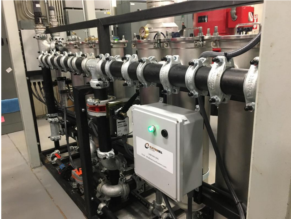
EC-6000 as installed
